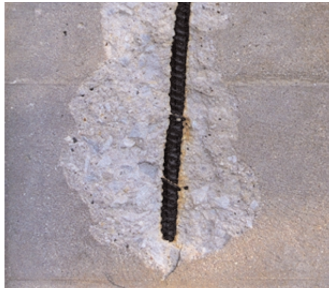
Fig. 1-29. Carbonation destroys concrete's ability to protect embedded steel from corrosion. All concrete carbonates to a small depth, but reinforcing steel must have adequate concrete cover to prevent carbonation from reaching the steel. This reinforcing bar in a wall had less than 10 mm (0.4 in.) of concrete cover; the ACI building code requires a minimum of 38 mm (1½ in.). After years of outdoor exposure, the concrete carbonated to the depth of the bar, allowing the steel to rust and spall the concrete surface. (68340)
