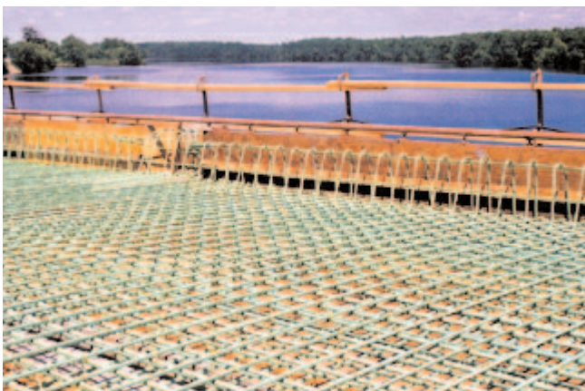
Fig. 1-30. Epoxy-coated reinforcing steel used in a bridge deck. (69915)
