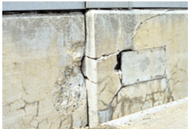
Fig. 1-27. Cracking, joint closing, spalling, and lateral offset are caused by severe alkali-silica reactivity in this parapet wall. (56586)
